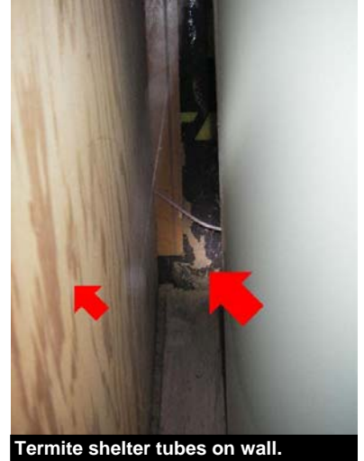
Termite shelter tubes on wall.
