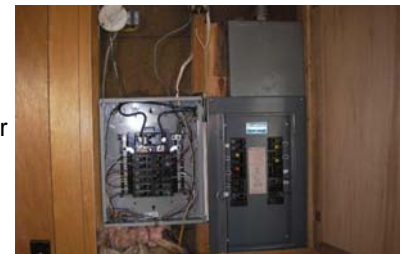
Wood paneling covers bottom of elec
