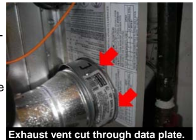
Exhaust vent cut through data plate.
